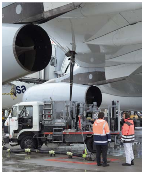
Meter Controller MFX_4 installed on Dispenser/Refueller
